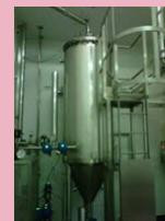
Bulk holding tank
